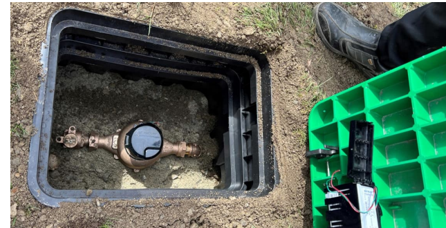
Accelerated metering program Implement AMI system & install 7,000 meters at unmetered properties (by 2027), $23M
