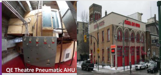
QE Theatre Pneumatic AHU
