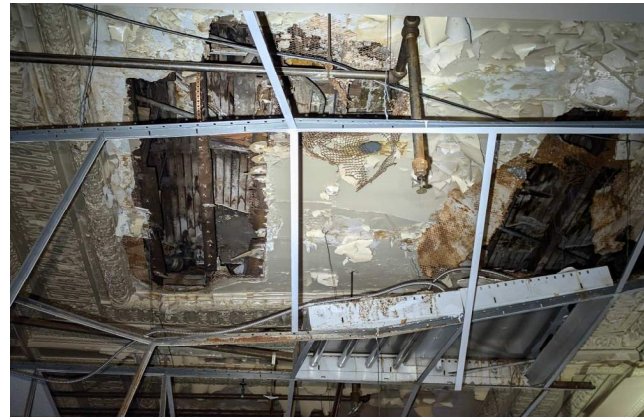
Figure 20, Main floor ceiling water ingress.
