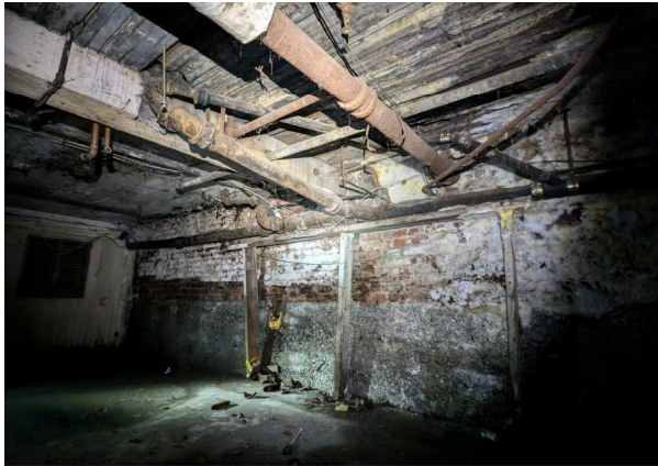
Figure 25, Floor rot, mold and compromised beam.
