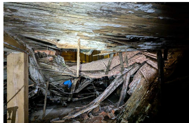
Figure 28, Collapsed floor, and rotten floor.
