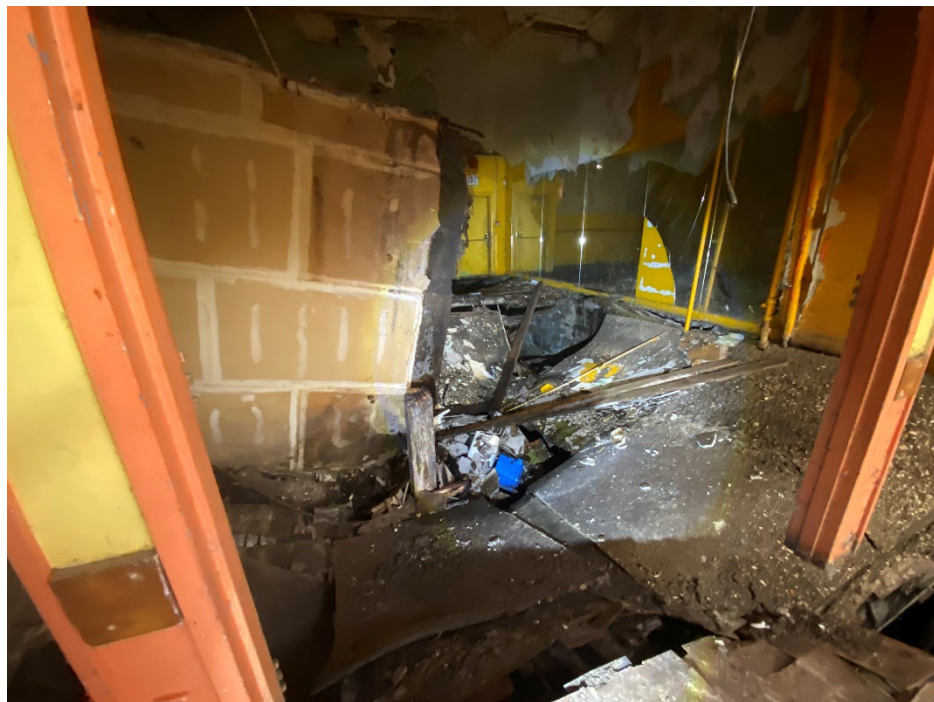
Ground floor collapsed into basement below SE skylight
