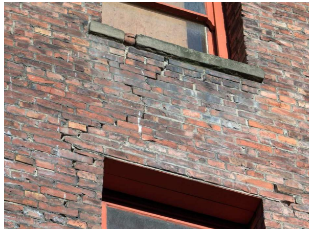
Figure 40, Diagonal shear cracks.
