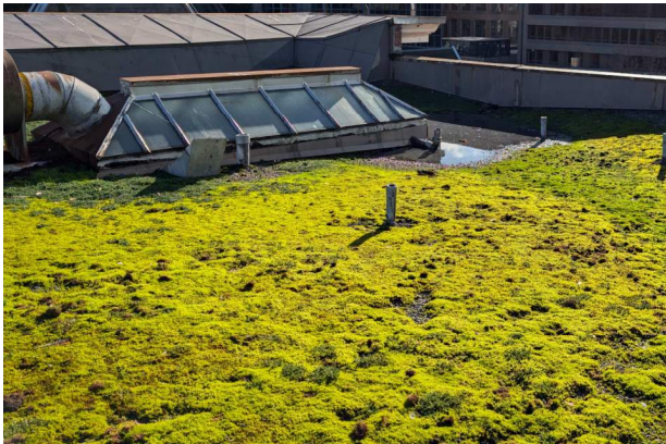
Figure 5, Southeast skylight with water ponding.
