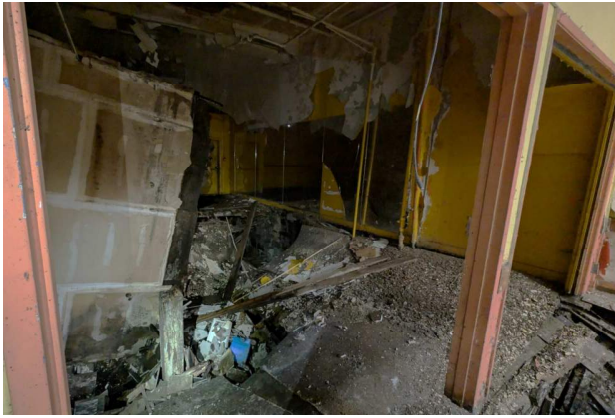
Figure 21, Complete floor structural collapse.
