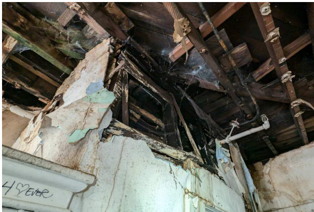
Figure 11, Buckled rotten wall under roof.
