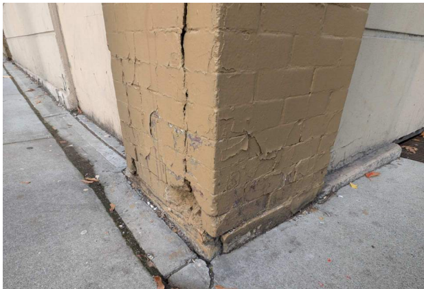
Figure 43, Cracking, spalling of column cladding.
