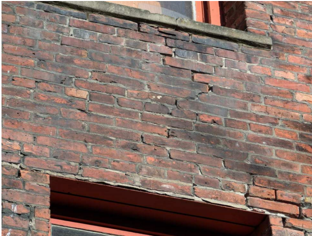
Figure 37, Vertical shear cracks and mortar loss.
