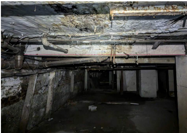
Figure 31, Deflection with red line for reference.
