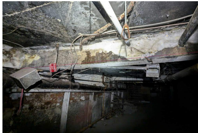
Figure 34, Deflection with red line for reference.
