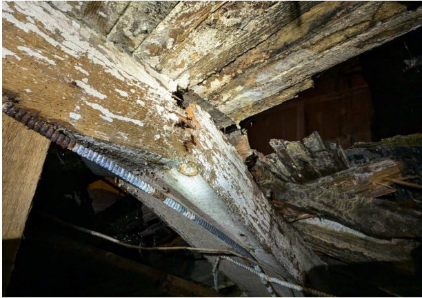
Figure 29, Fully failed rotten beam.
