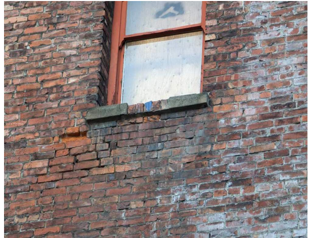
Figure 38, Mortar loss and degraded brick.
