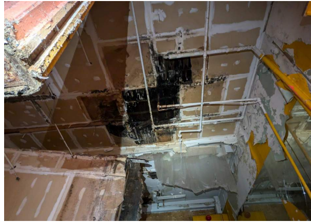
Figure 30, 2 nd floor rot as seen from the basement.
