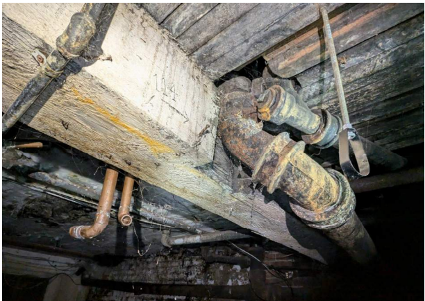
Figure 33, Failed beam due to side notch for pipe.
