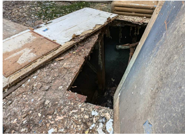
Figure 24, Localized floor collapse.
