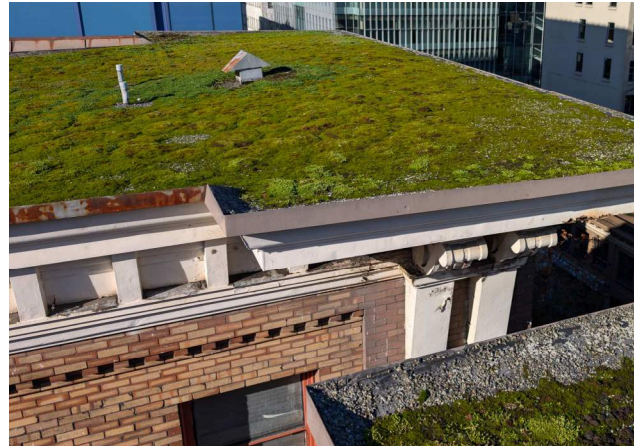
Figure 4, Roof with moss growth and cornice.
