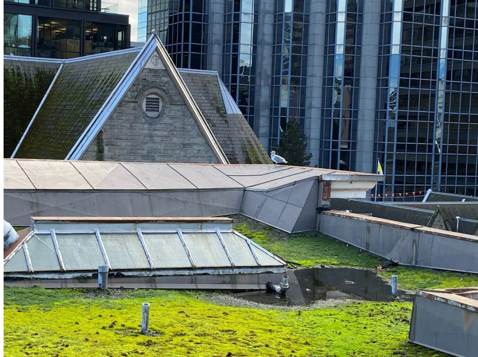
Water ponding on roof near SE skylight
