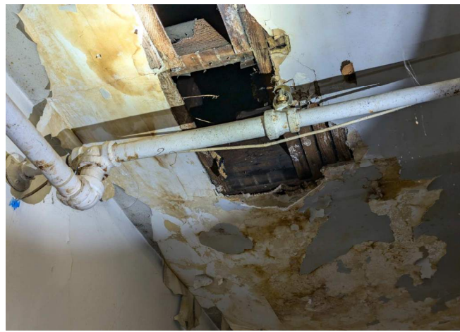
Figure 8, Top floor ceiling, north end hallway.
