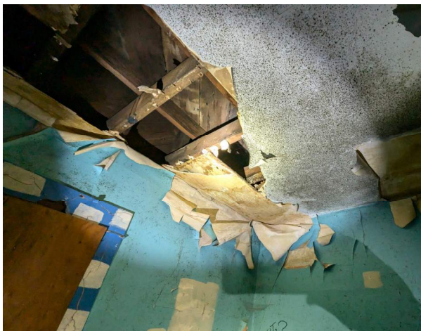
Figure 7, Top floor ceiling, north end hallway.
