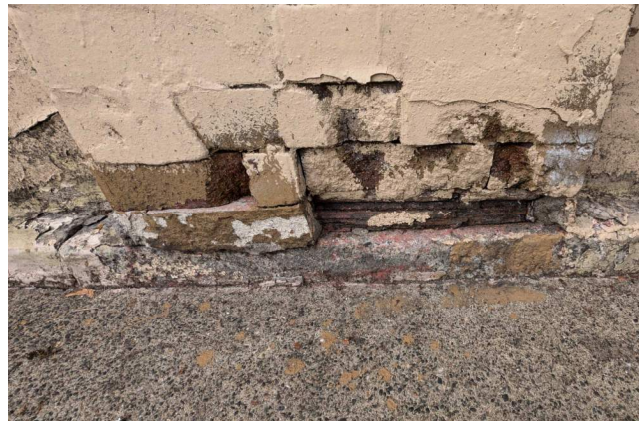
Figure 44, Steel column baseplate exposed & rusting.
