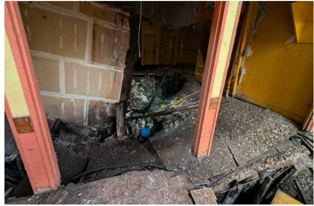
Figure 22, Complete floor structural collapse.
