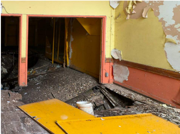
Figure 23, Complete floor structural collapse.
