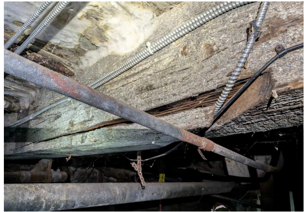
Figure 32, Failed beam due to notch for wire.
