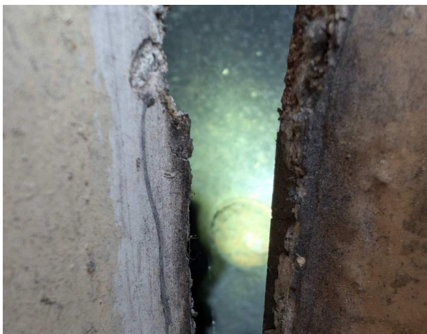
Figure 45, Rivet of steel column seen through crack.
