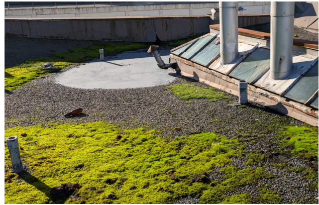
Figure 6, Southwest skylight with water ponding.
