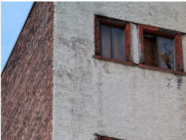
Figure 41, Vertical interface cracks.
