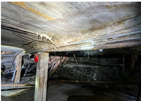
Figure 27, Floor rot, beam rot and mold.
