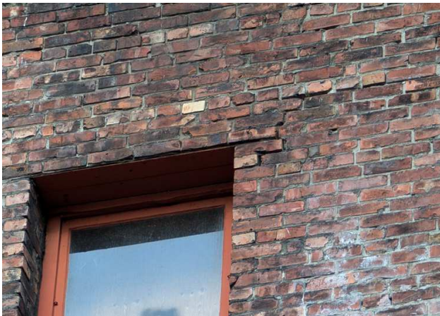
Figure 39, Diagonal shear cracks.
