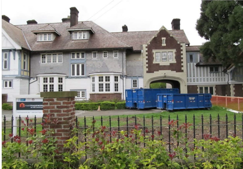
Figure 6 Rosemary, 3689 Selkirk Street, 2015. View from the front yard of the ongoing refurbishment of the exterior cladding.
