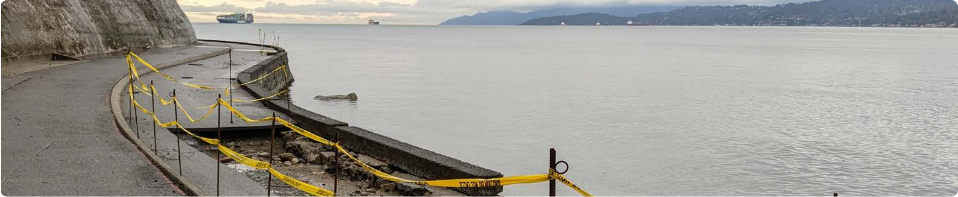
▲ Damage to the Stanley Park seawall following king tides and stormy weather (Source: Vancouver Park Board)
