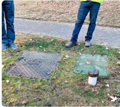
▼ Staff inspect a new park water meter (Source: City of Vancouver)
