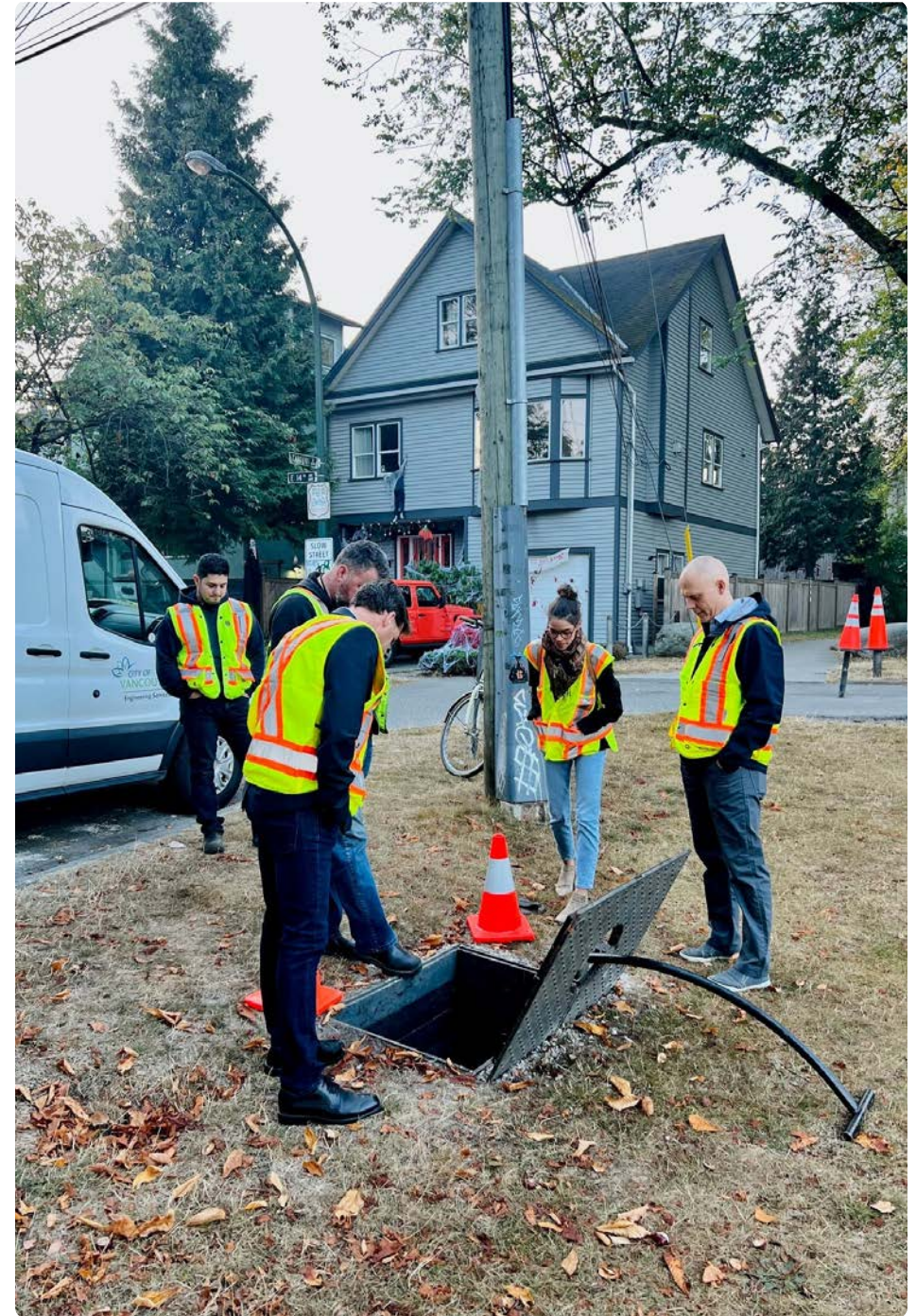
Staff inspect a new park water meter that resulted in locating a leak for repair (Source: City of Vancouver) ►
