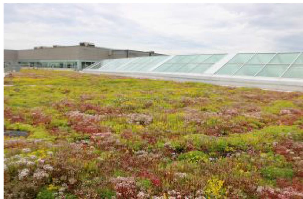
Sedum Greenroof Supplier: Next Level stormwater management
