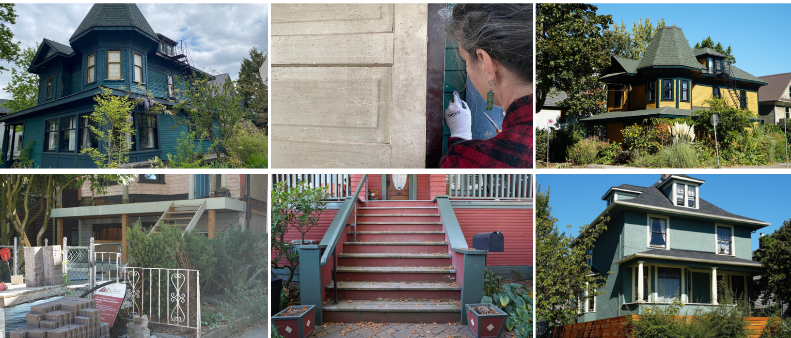
L to R Top: True Colours Painting Before, True Colours Paint Scraping, True Colours Painting After (Photos: E.Y. Pan, M. Lenz/VHF) L to R Bottom: Foundation Repairs; Porch Repairs; True Colours Painting (Photos: E.Y. Pan)
