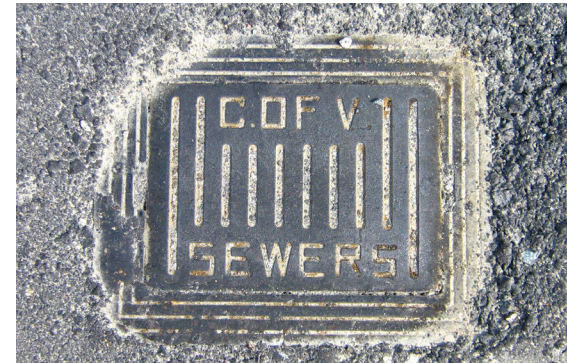
Sewer cleanout box cover
