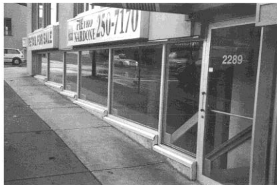
Figure 5. Example of undesirable response to topography - basement spaces
