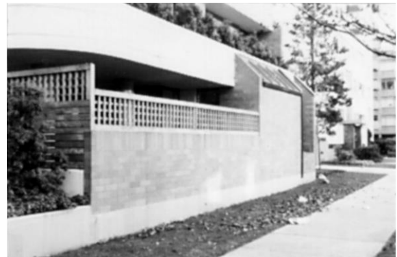
A high blank, wall along the street edge creates an inhospitable image.
