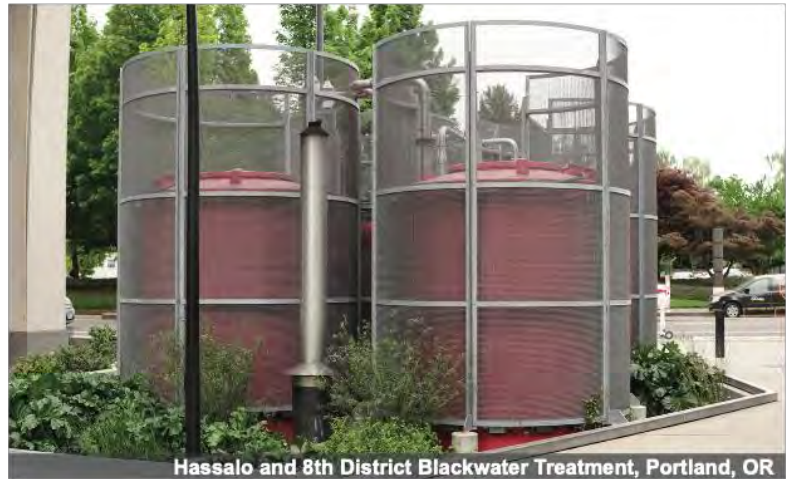
Hassalo and 8th District Blackwater Treatment, Portland, OR
