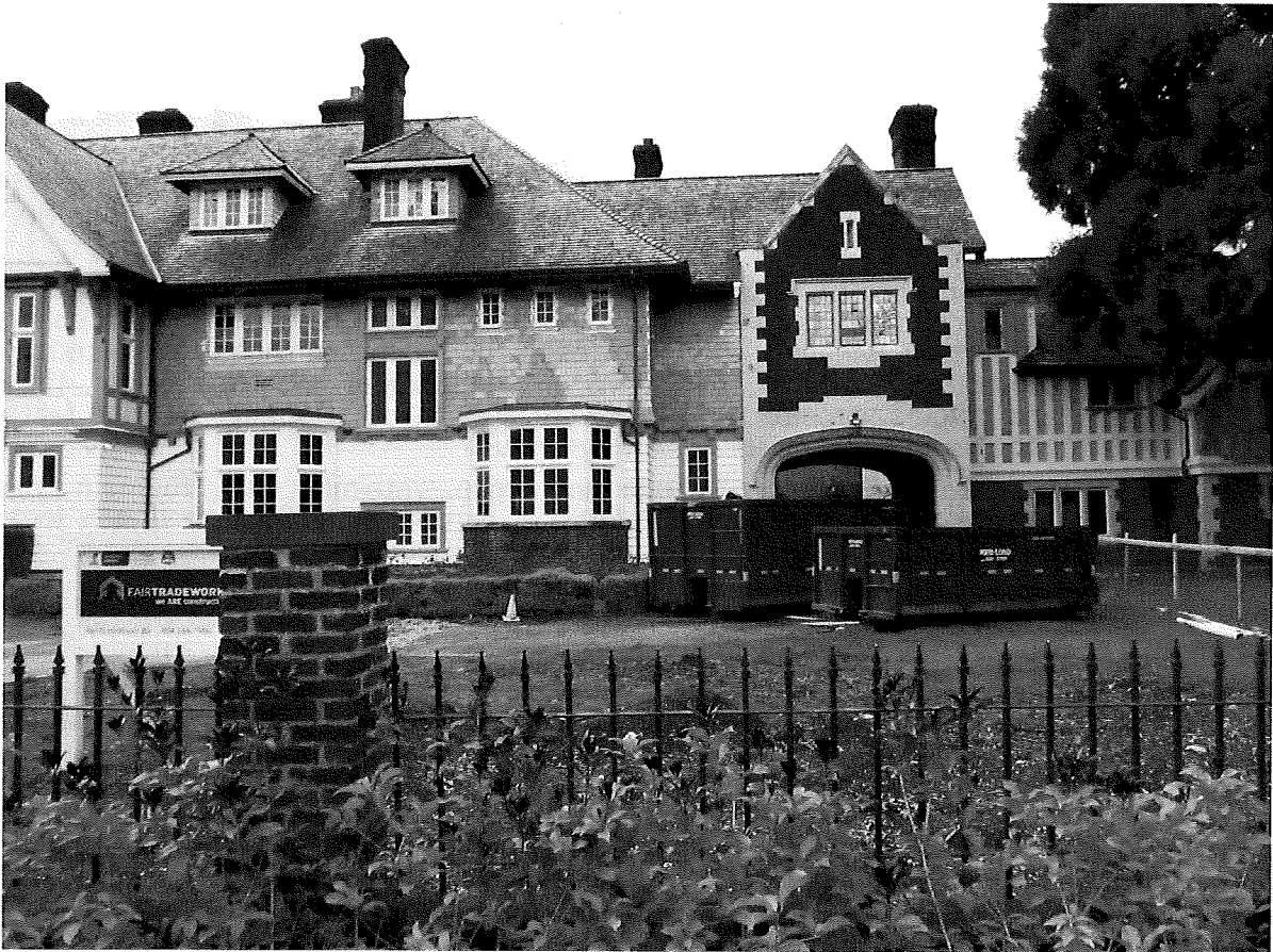
Above: Rosemary, 3689 Selkirk Street, 2015. View from the front yard of the ongoing refurbishment of the exterior cladding.
