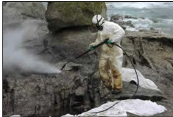
Clean-up following Prestige spill. (Source: ITOPF)
