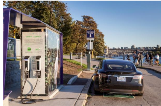
Electric vehicle charging station in English Bay Beach Park.
