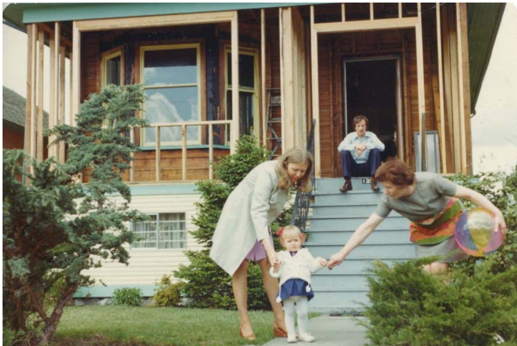
Photo 4: filling in the porch circa early 1960s (photo courtesy of the Wegner family). The photographs from the Wegner family were invaluable in assessing the restoration strategy and the changes which had occurred over time.
