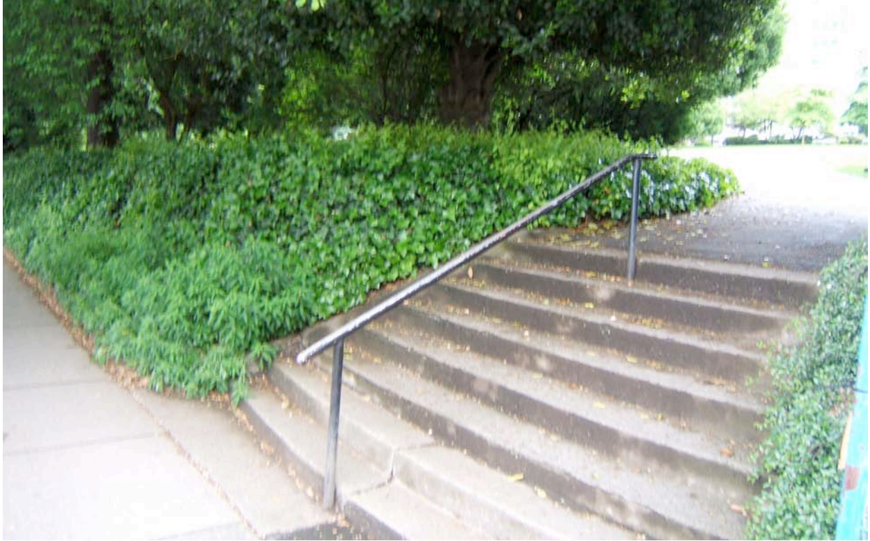
EXISTING STAIRS AT CAMBIE AND 10th To be replaced with new stairs with Art Deco detailing.
