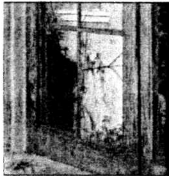
Photo 29: Desiccated windows requiring maintenance
