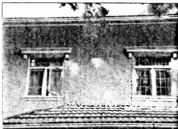
Section of original stucco to be preserved in situ as an archival record, south elevation between WUS3 and WUS4
