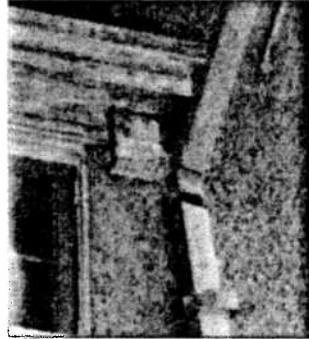
Photo 25: Poorly-maintained downspout where junction has been broken
