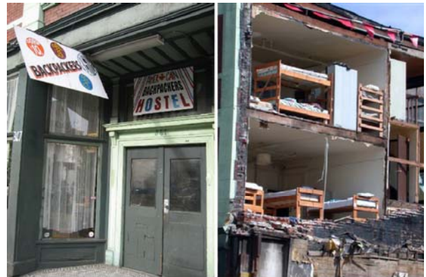
NEW BACKPACKERS HOSTEL - ENTRANCE - SIDE WALL AFTER DEMO OF BLDG. NEXT DOOR
