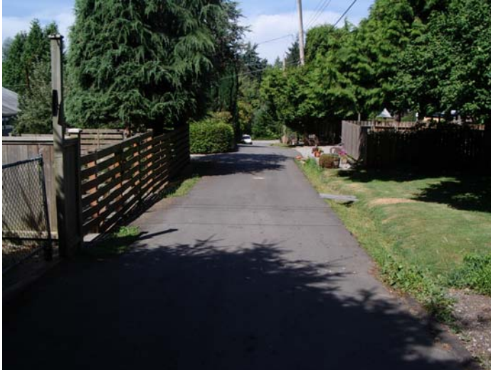
Photograph of District of North Vancouver's Low Cost Center Strip Lane Paving
