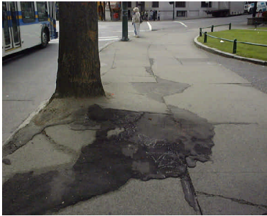
root damage to sidewalk
