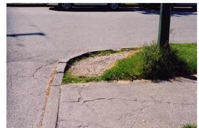
increasing sidewalk problems
