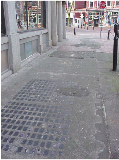
black asphalt is a poor repair solution
