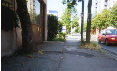
tree root damage can be extensive
