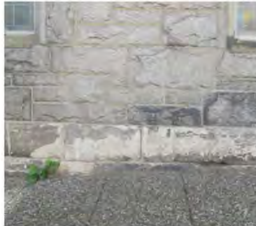
Above grade vegetation and damaged sandstone growth
