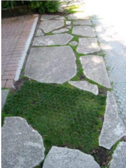
Figure 5.7 Broken Concrete Driveway Connections
